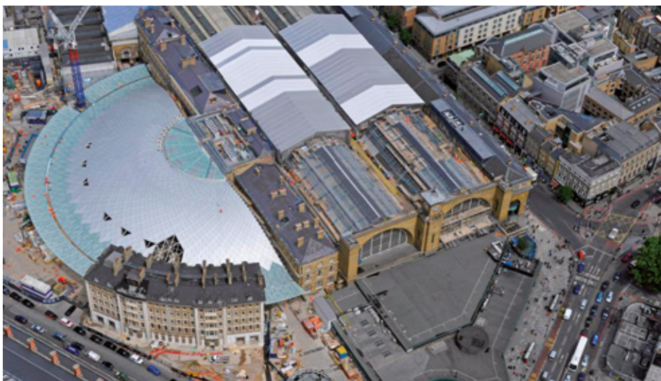
Powerclad Keder Roof Sheeting on Kings Cross Station – Europe's largest temporary roof structure
